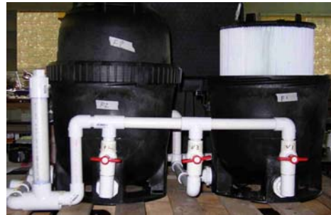
Pre-filters showing cartridge and valves
